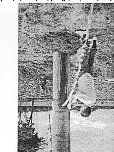
Piezometric tube not yet fixed to airtvent standpipe SP 33096 Saherber Gaon, Sunamganj
