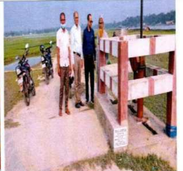
Regulator (1 Vent) of Balia Bhangunkul Subproject, Tala, Satkhira.
