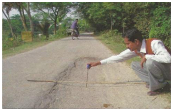
Figure 2-9 Need for routine pavement maintenance
