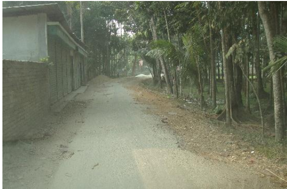
Damaged surface & shoulder of a Laksmipur Road, awaiting improvement under UGIIP III
