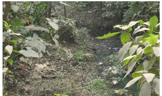
A major Lakhipur primary drain – overgrown with vegetation, which impedes timely drainage
