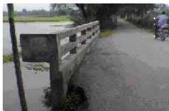
Figure 9: Damaged culverts & approaches were reconstructed
