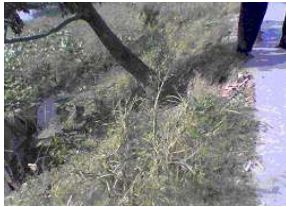
Figure 1: Slope and shoulder damaged due to the failure of Palisade
