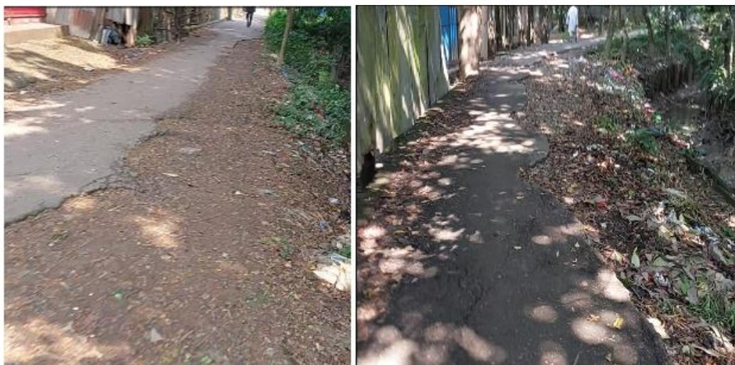
Existing Road Condition at Sheikh Para Primary School Road
