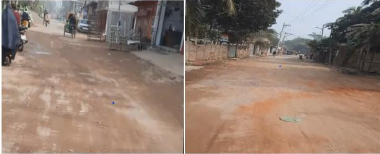
Photographs: Existing Road Condition starting from Hazi More to Katarpul of the Subproject Site
