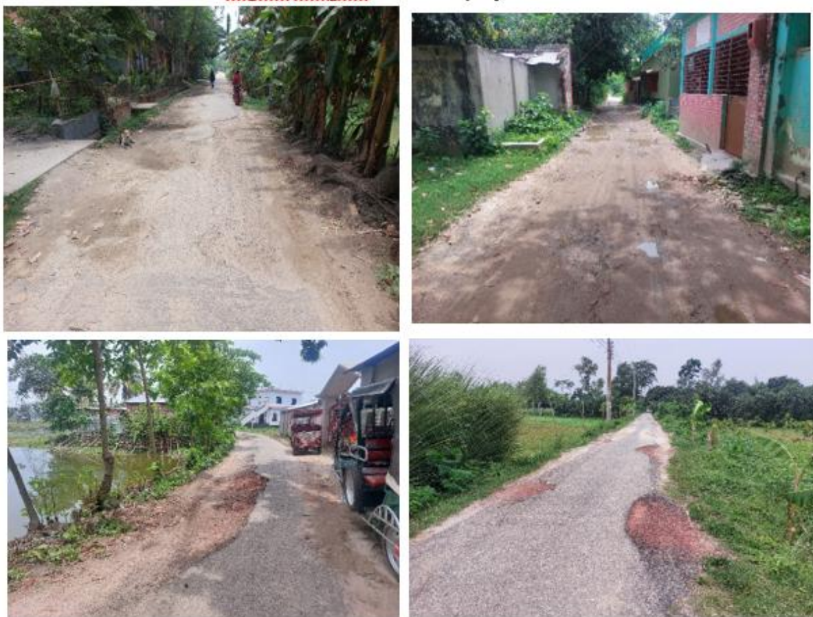
Photograph 2.2.2: Existing Road Condition from Gulshanmore to Kutibari Bridge via- Khaonjjonpur Registry Office of the Subproject Site
