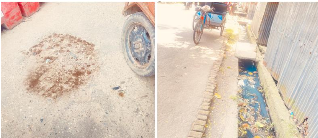
Photograph 2.2.2: Existing road and Drain Condition at Sher-e Bangla Road (Patch Matha Mor to Gol Chattar) of the Subproject Site
