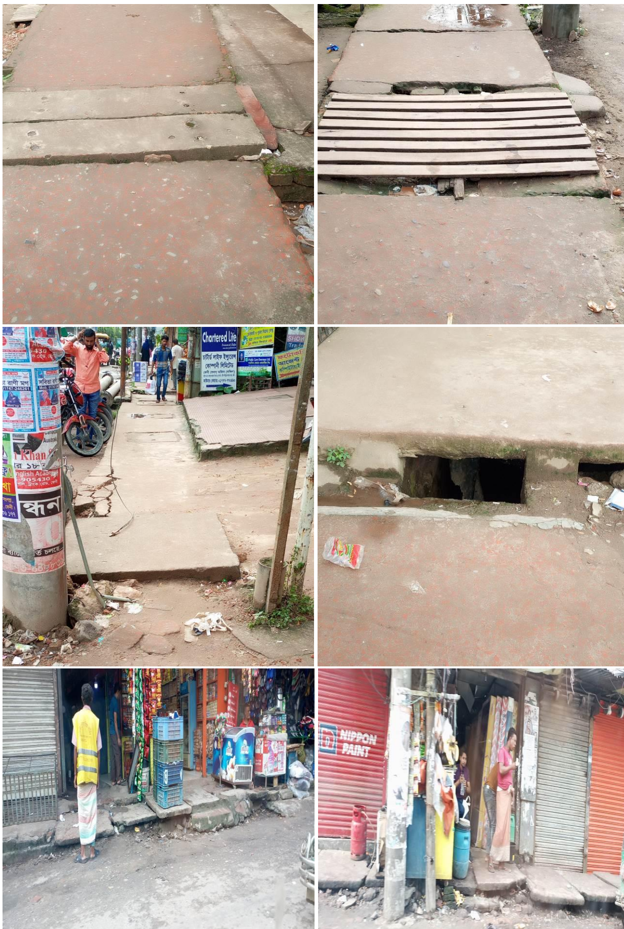
Photographs 2.2.1(a): Existing Drain Condition at Shaheed Shahidullah Kaiser Road (Feni trunk road to Mohipal Zero point) of the Subproject Site
