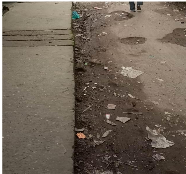
Photographs 2.2.1(e): Existing Drain Condition at Art Academy Road of the Subproject Site
