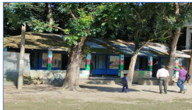
Figure 7: Tin shed building needs to be demolished
