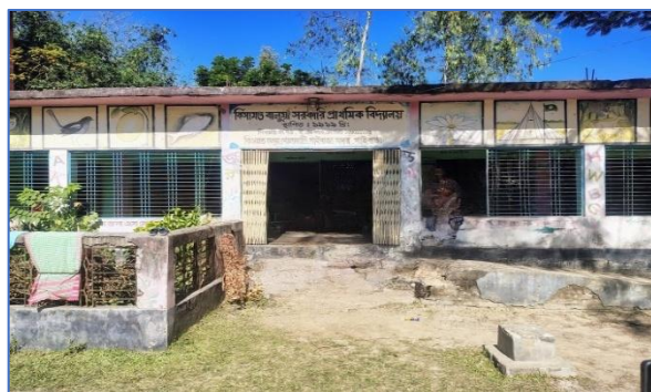
Figure 7: The Old School Building needs to be Demolished
