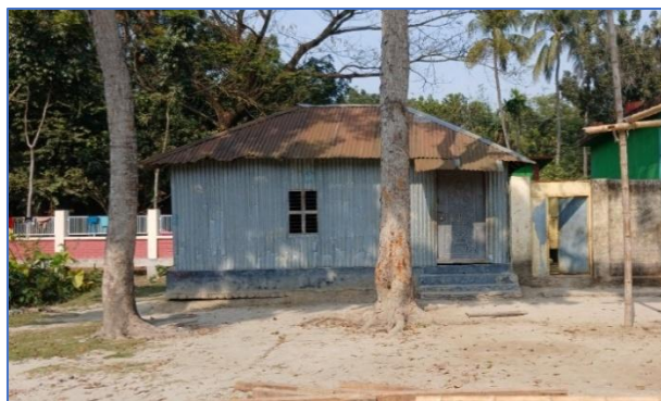
Figure 8: Tin-Shed School Need to be Demolish
