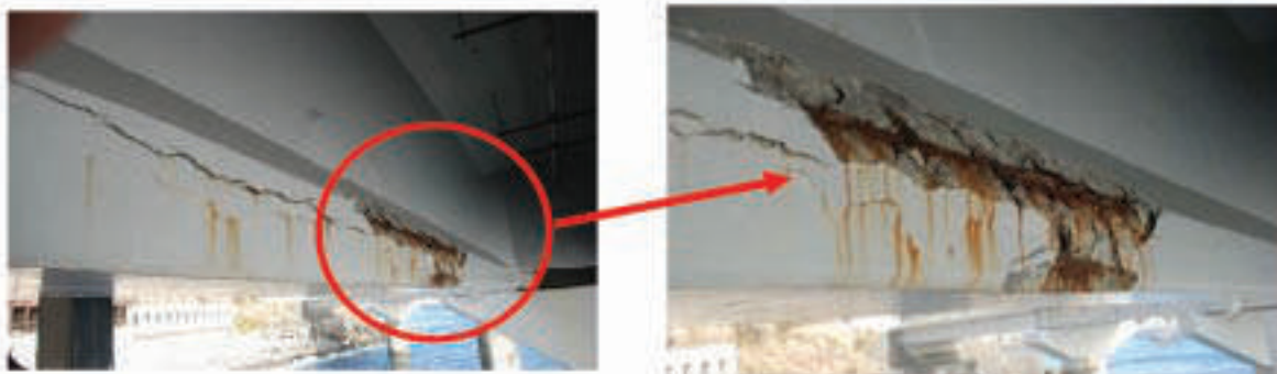
Spalling, Exposed rebar by chloride attack
