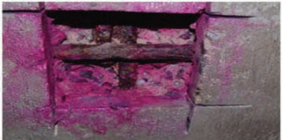
Photo-7.7.7 Phenolphthalein method by exposed rebar and Rebar corrosion
