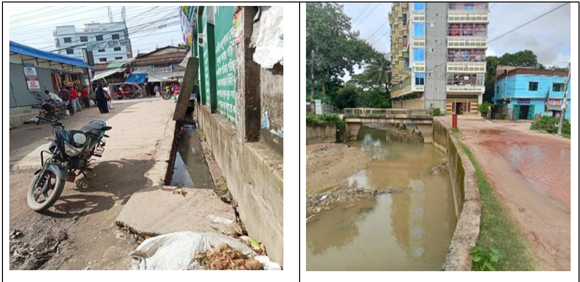
Photograph 2.2.2: Current Situation of the Drain and Outfall at Subproject Site
