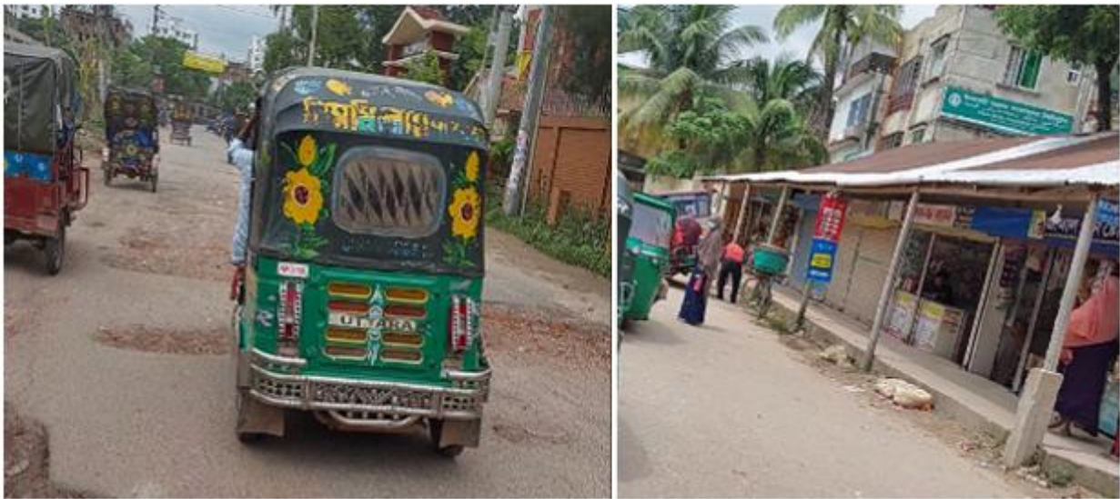
Photographs 2.2.1(b): Existing Road Condition at Noakhali Sadar Hospital Road of the Subproject Site
