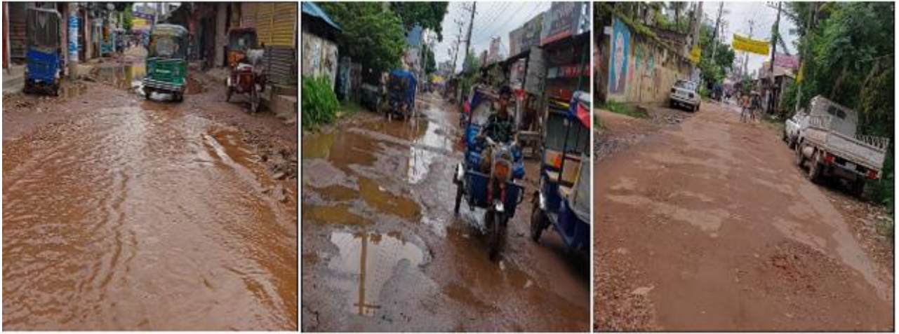
Photographs 2.2.1(a): Existing Road Condition at at Majdee New Jail Road of the Subproject Site
