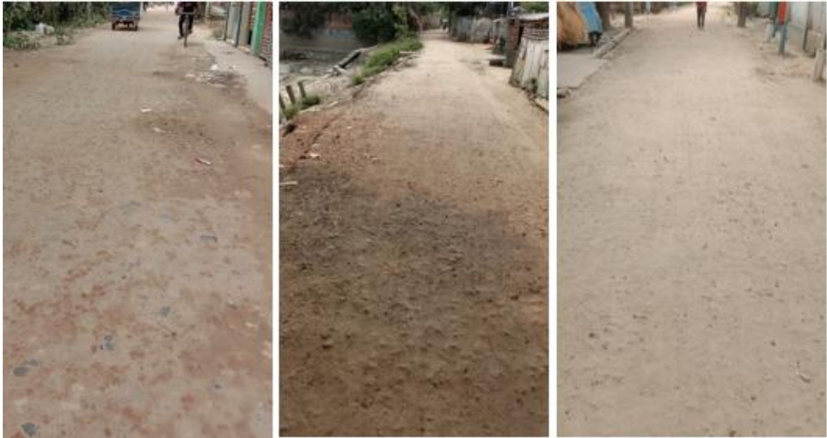
Photographs 2.2.1: Existing Drain Condition of the Subproject Site
