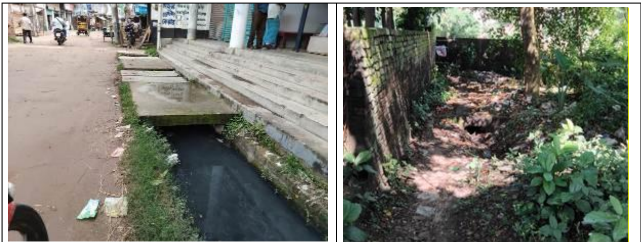
Photograph 2.2.2: Current Situation of the Drain and outfall at Subproject Site
