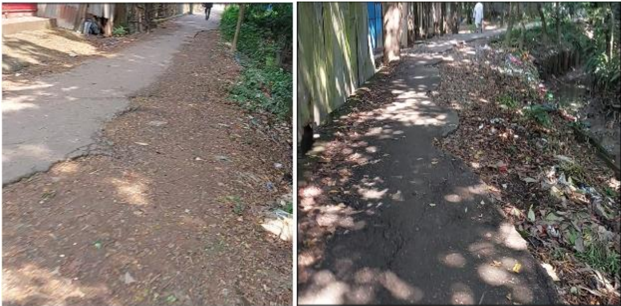
Photographs 2.2.1: Existing Road Condition at Sheikh Para Primary School Road
