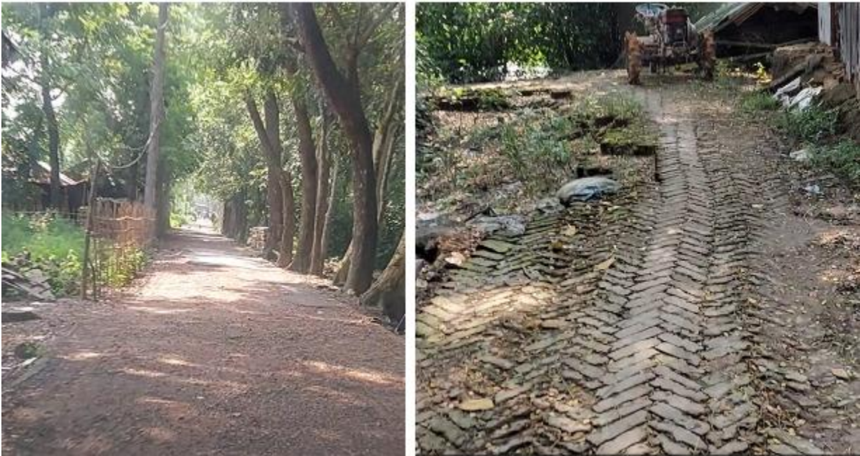
Photographs 2.2.2: Existing Road Condition at Amir Hosain Miazi Road
