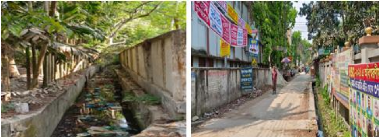
Photographs 2.2.2: Existing Drain Condition of the Subproject Site
