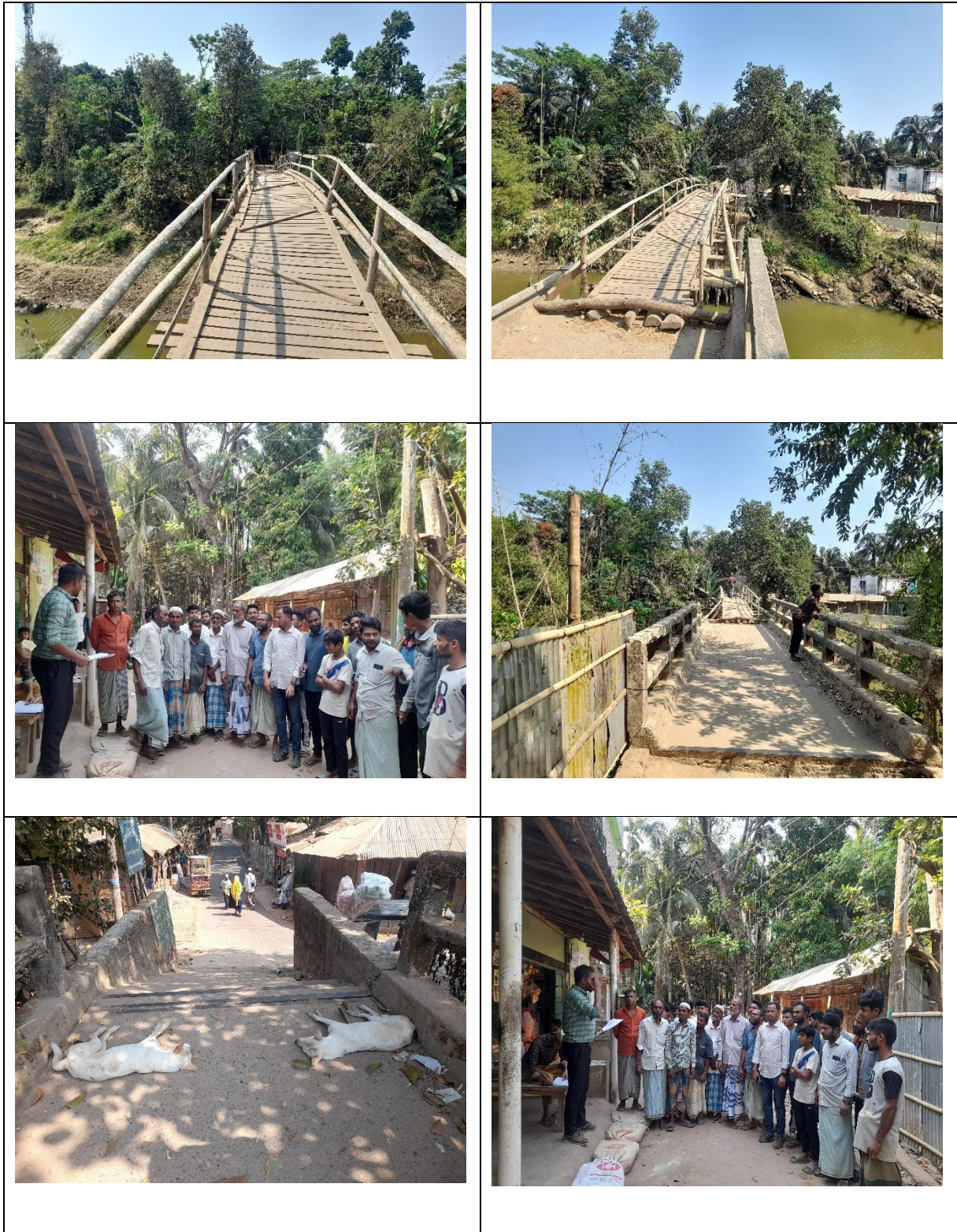
Figure: Present condition of the proposed location for 57m Long RCC Bridge on Eidgaon GC atMaijpara - Pokkhali (Faraze Para Road) at Ch. 2350m, Sadar Upazila District: Cox's Bazar, Road ID- 422243002
